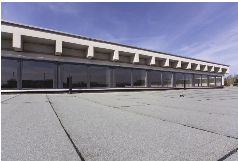
The roof of the secondary modern school after energy-related renovation. Source: Vedag GmbH
