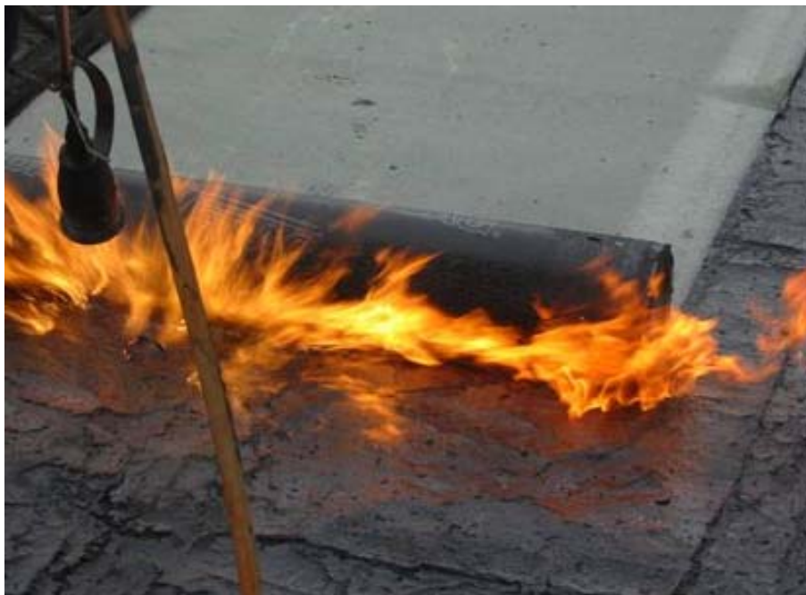
The first layer (VEDAFLEX G4E) is applied to the prepared surface. Source: VEDAG GmbH
