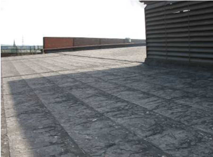
The poor condition of the roof of the Georgsmarienhütte before the revitalisation. Source: VEDAG GmbH
